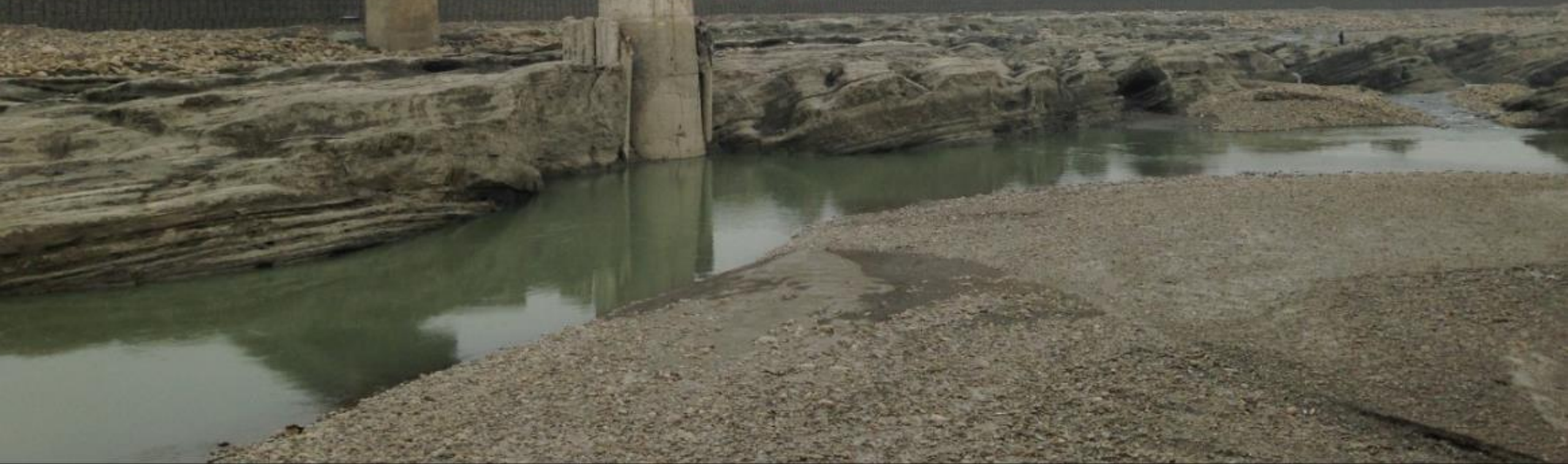
Bedrock Erosion With Bridge Failure (Tou-Chien River, Taiwan, Chung-Ta Liao 2014)
