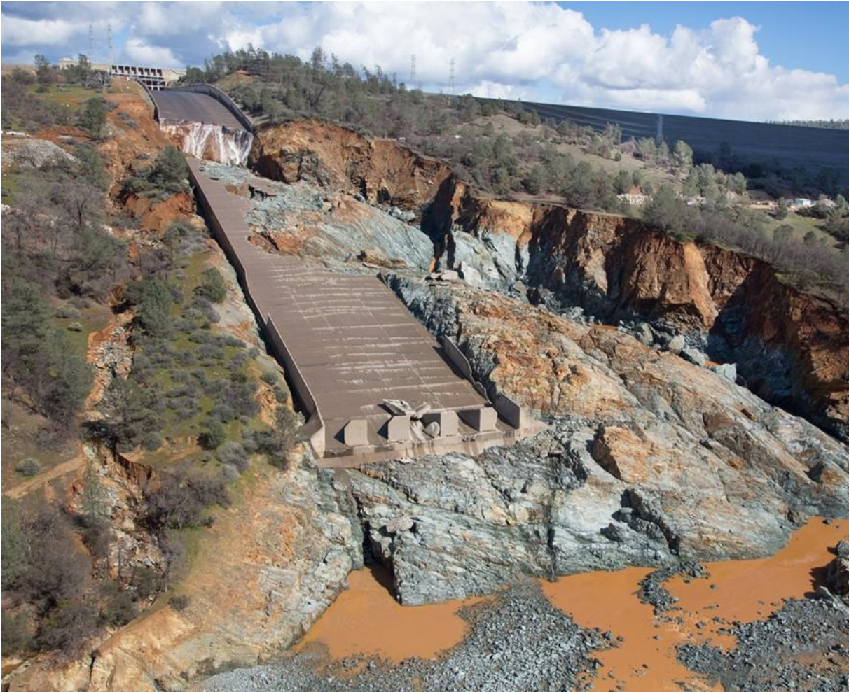
Figure 10. Oroville dam spillway failure (LA Times)
